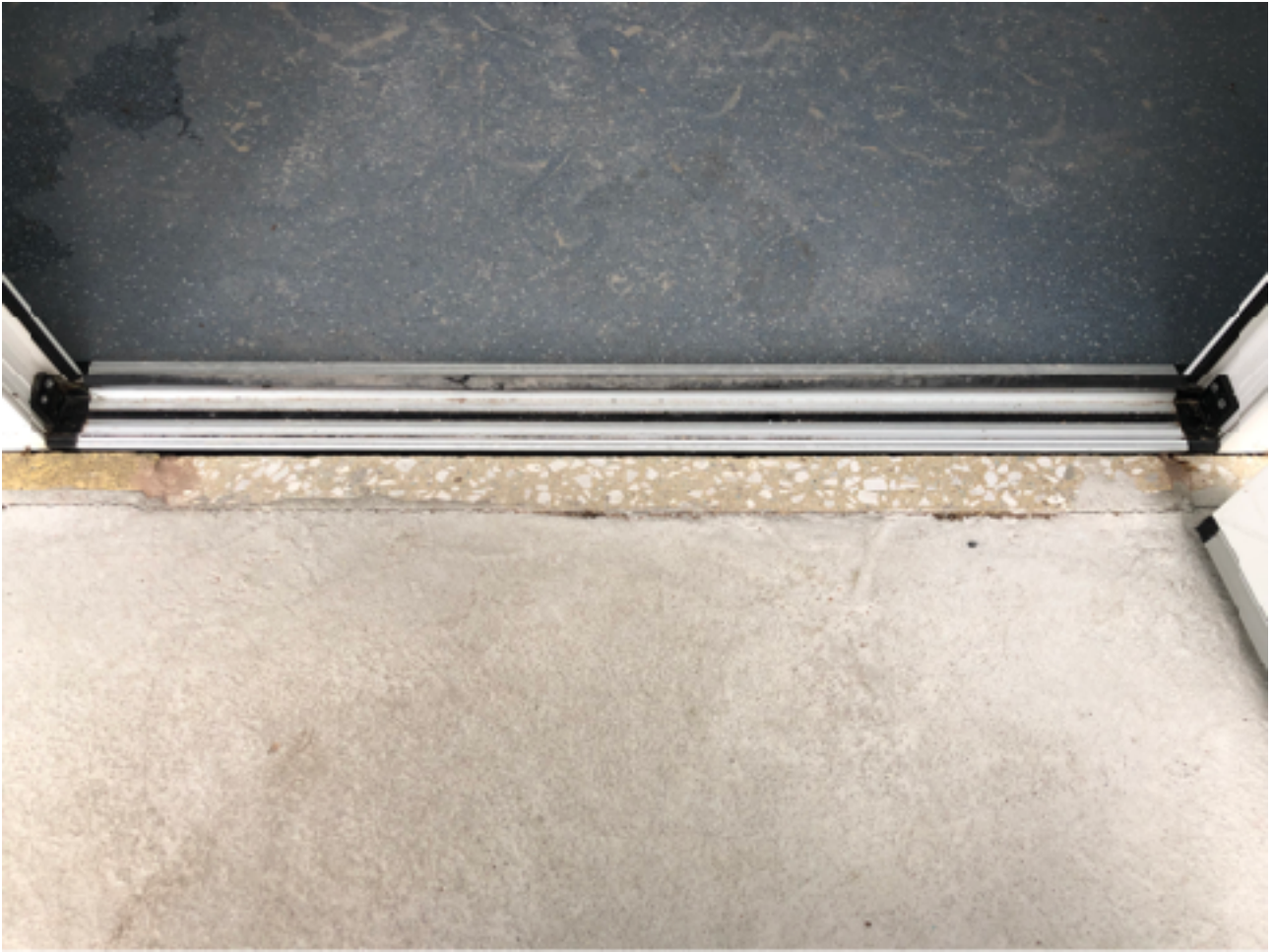
[Picture of disabled toilet/shower unit door threshold]
